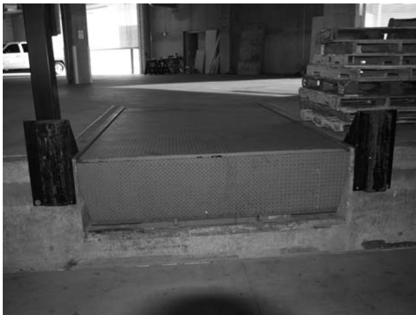
FIGURE 35.3 Dock leveler. (Photo by author, courtesy of The University of Southern California.)
