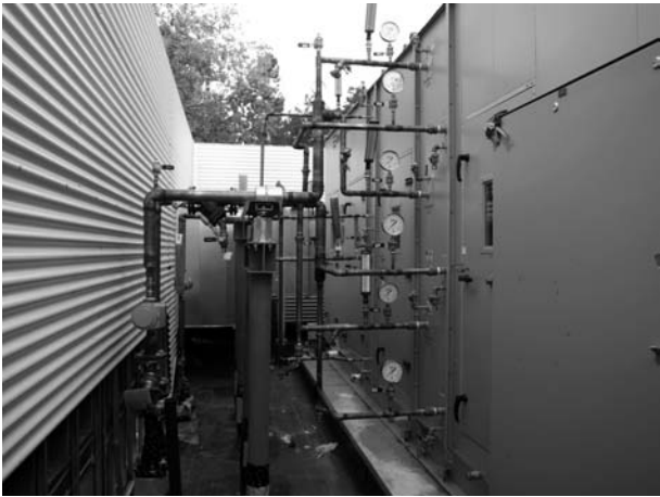
FIGURE 40.2 Hydronic piping at an air handling unit (AHU). (Photo by author, courtesy of Hathaway Dinwiddie Construction Company and California State University Northridge.)
