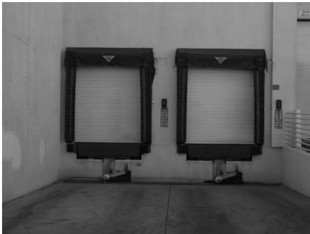
FIGURE 35.4 Dock seals and bumpers.
