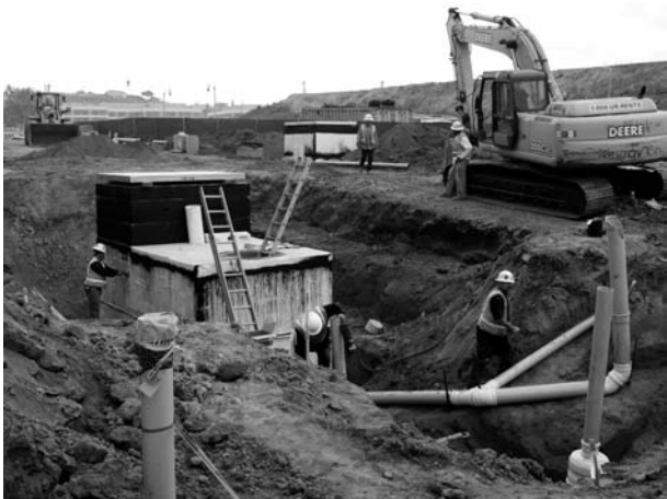
FIGURE 42.2 In-ground vault. (Photo by author, courtesy of Hathaway Dinwiddie Construction Company and Tishman Speyer.)
