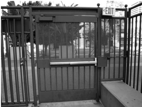
FIGURE 12.6 Door hardware at metal gate.
