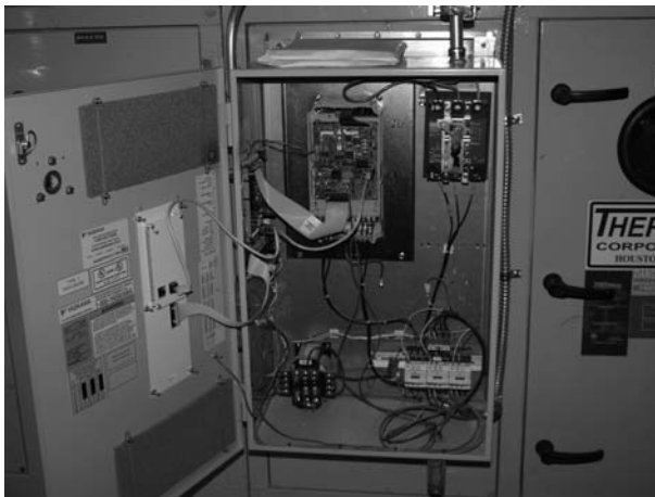
FIGURE 40.6 Variable frequency drive (VFD). (Photo by author, courtesy of Hathaway Dinwiddie Construction Company and The California Institute of Technology.)
