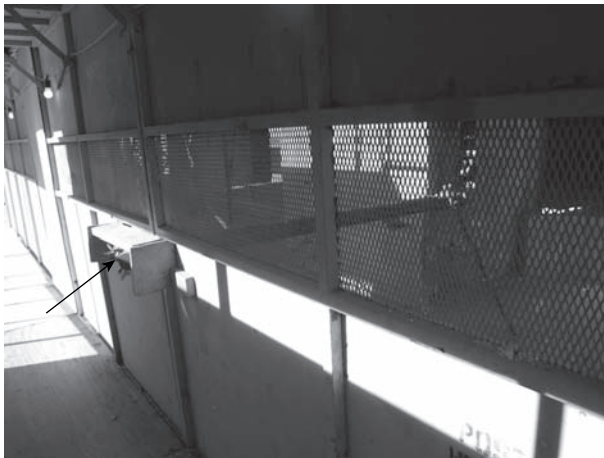
FIGURE 39.5 Temporary fire department connection.
