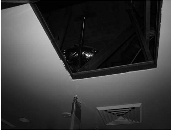
FIGURE 35.1 Ceiling mounted toilet partition. (Photo by author, courtesy of Hathaway Dinwiddie Construction Company and The California Institute of Technology.)
