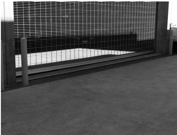
FIGURE 27.3 Coiling grille with heavy bottom bar. (Photo by author, courtesy of The University of Southern California.)
