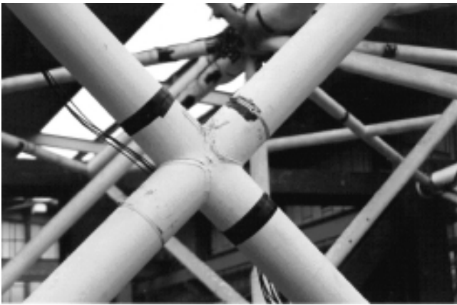
FIGURE 12.22 Tearing in tubular joint.
