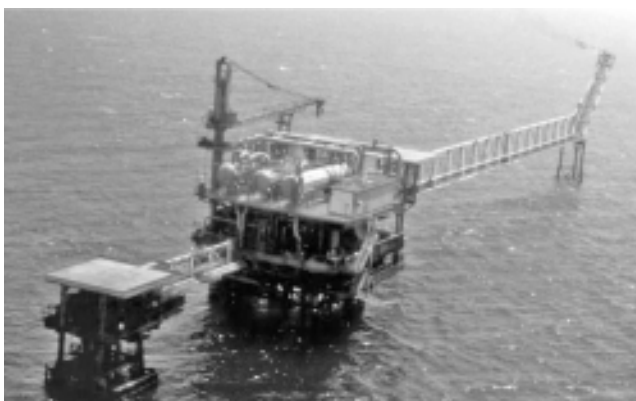
FIGURE 12.1 Production platform with bridges.
