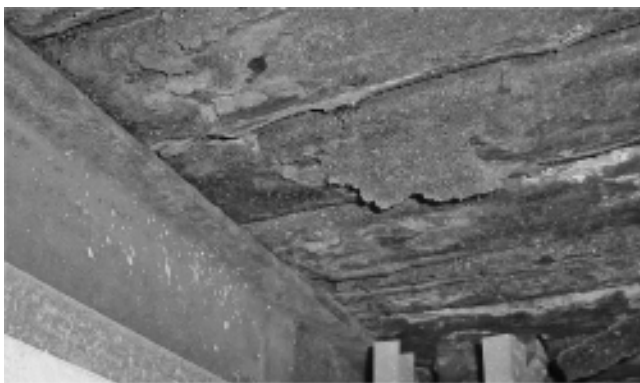
FIGURE 8.12 Corrosion in a corrugated sheet.
