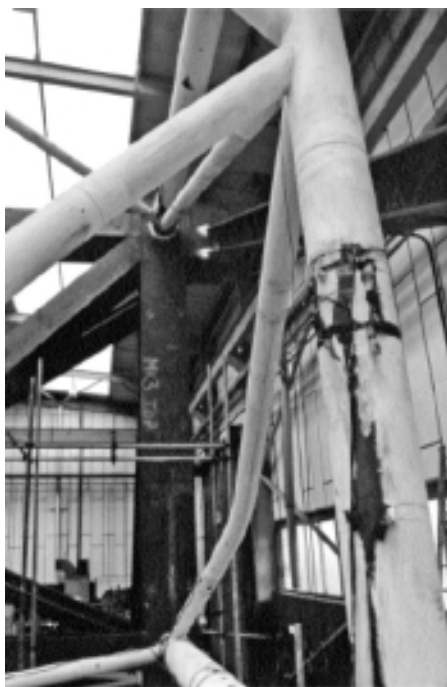
FIGURE 12.15 Buckling in a member for K bracing.
