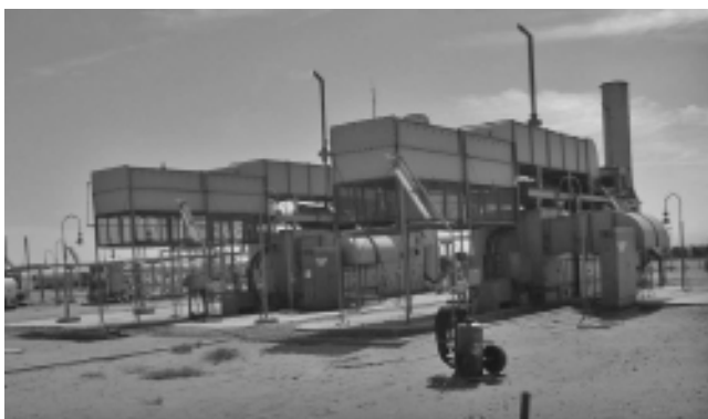
FIGURE 4.2 Gas turbine generator.
