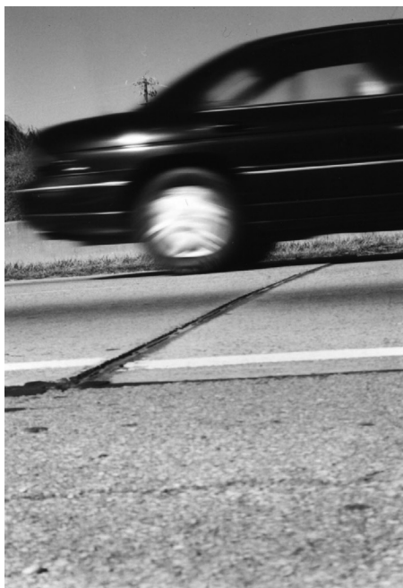
Figure 4.10 Faulted transverse joint. (Photo by author.)
